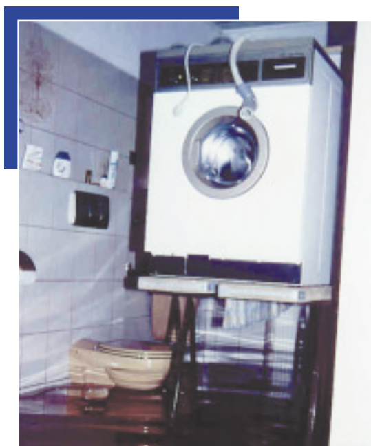
Elevating electrical equipment
