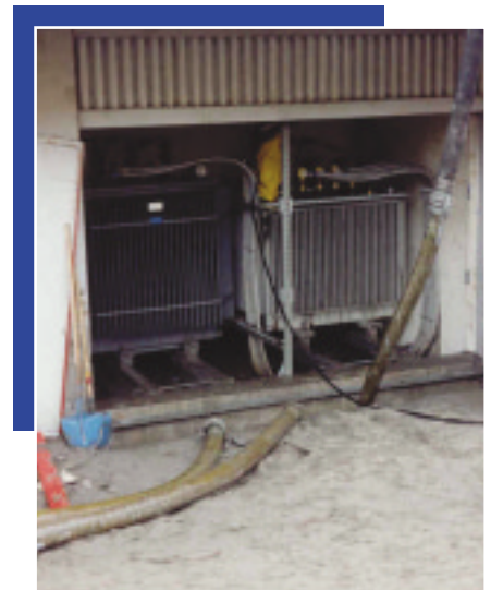
Damage due to dirt
