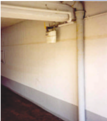
Elevated gas supply installation
