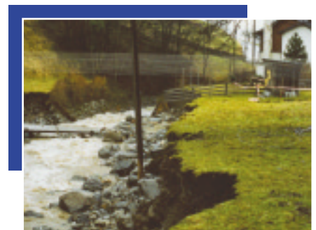
River bank erosion
