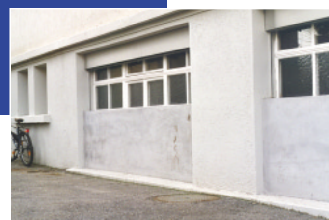
Sealing openings (permanently) by water resistant walls
