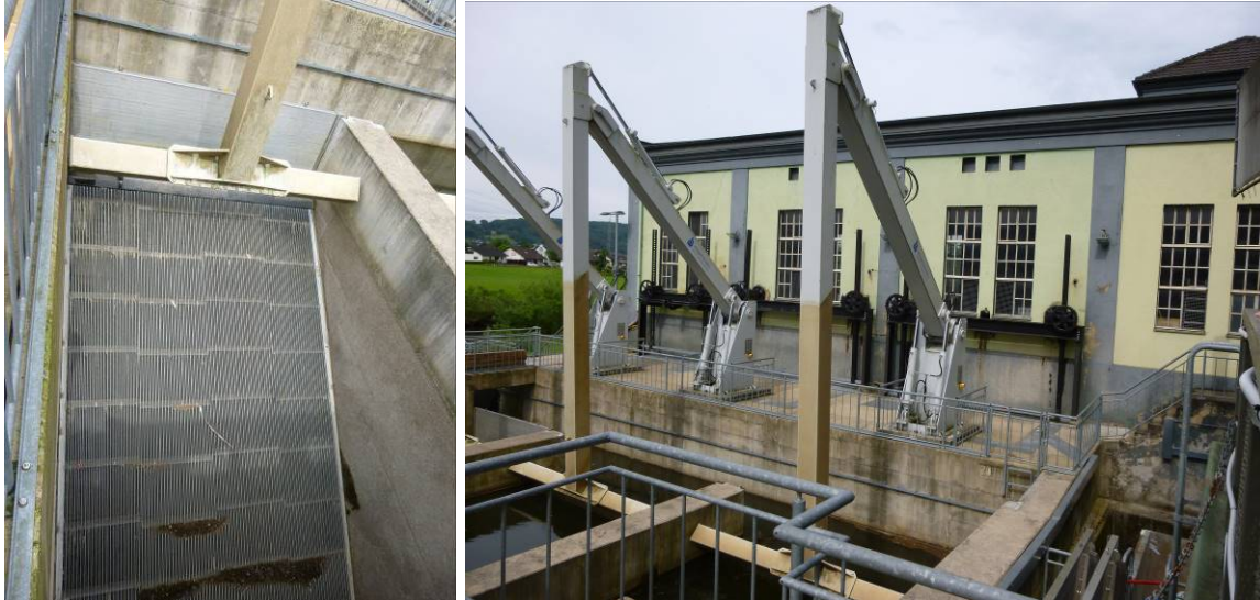
Figure 9. Vertical rake (10 mm) of the fish descent system at the Unkelmühle hydropower plant.
